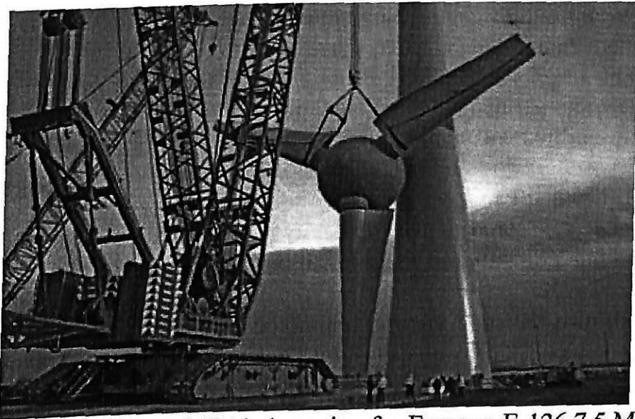
Figure 3.7- Lifting of the 340 t hub section for Enercon E-126 7,5 MW wind turbine. The Terex Demag CC9800 crawler crane is formally rated 1600 t and in this configuration can lift 360 t
