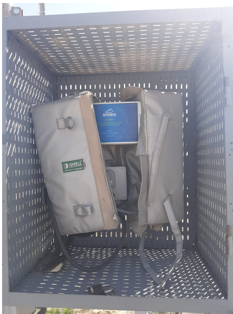
Figure 3.4 – View inside of sampling system box
